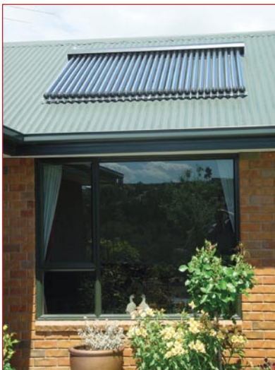
Figure 3: An evacuated tube collector installation
