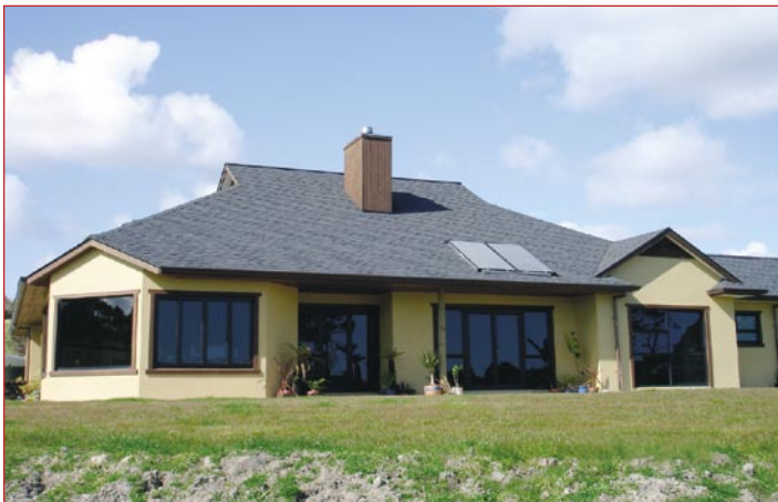
Figure 1: A flat plate collector installation
