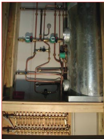
Figure 5: Solar heated cylinder with heat pump backup heating for underfloor heating system
